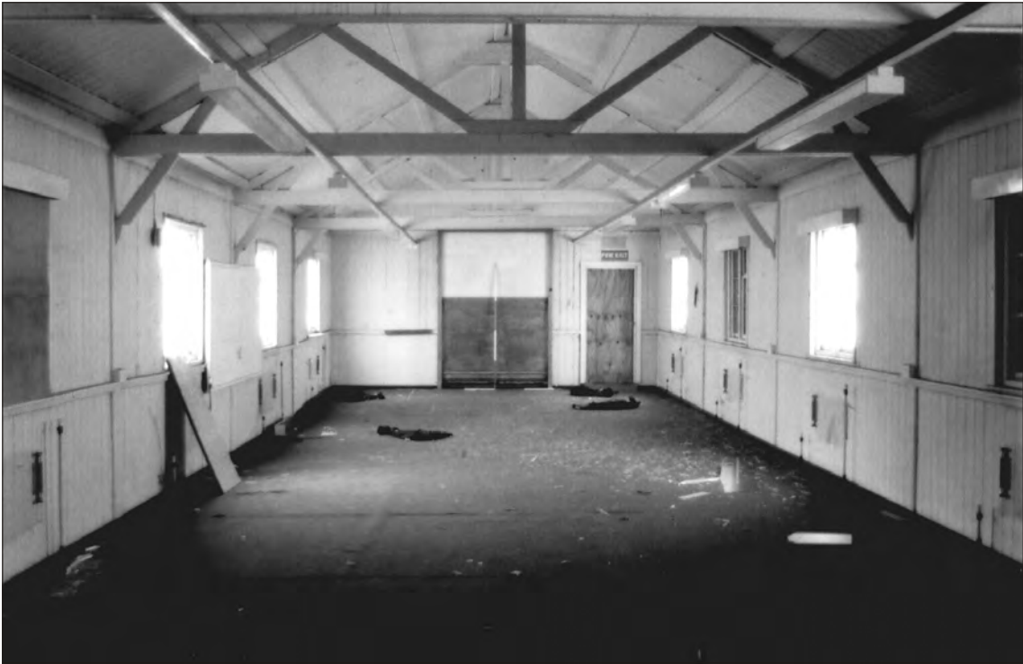
Plate 45 Saighton Camp, Chester: internal view of north-eastern 'leg' of building 39 looking north
