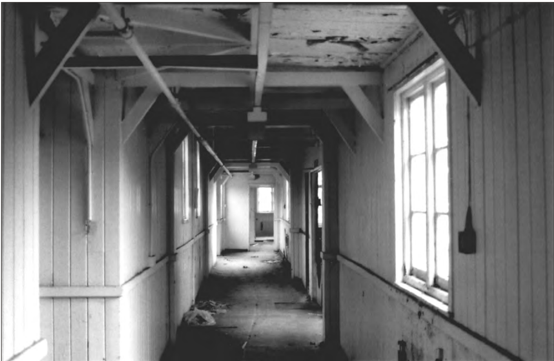
Plate 46 Saighton Camp, Chester: internal view of northernmost corridor of building 39, looking west
