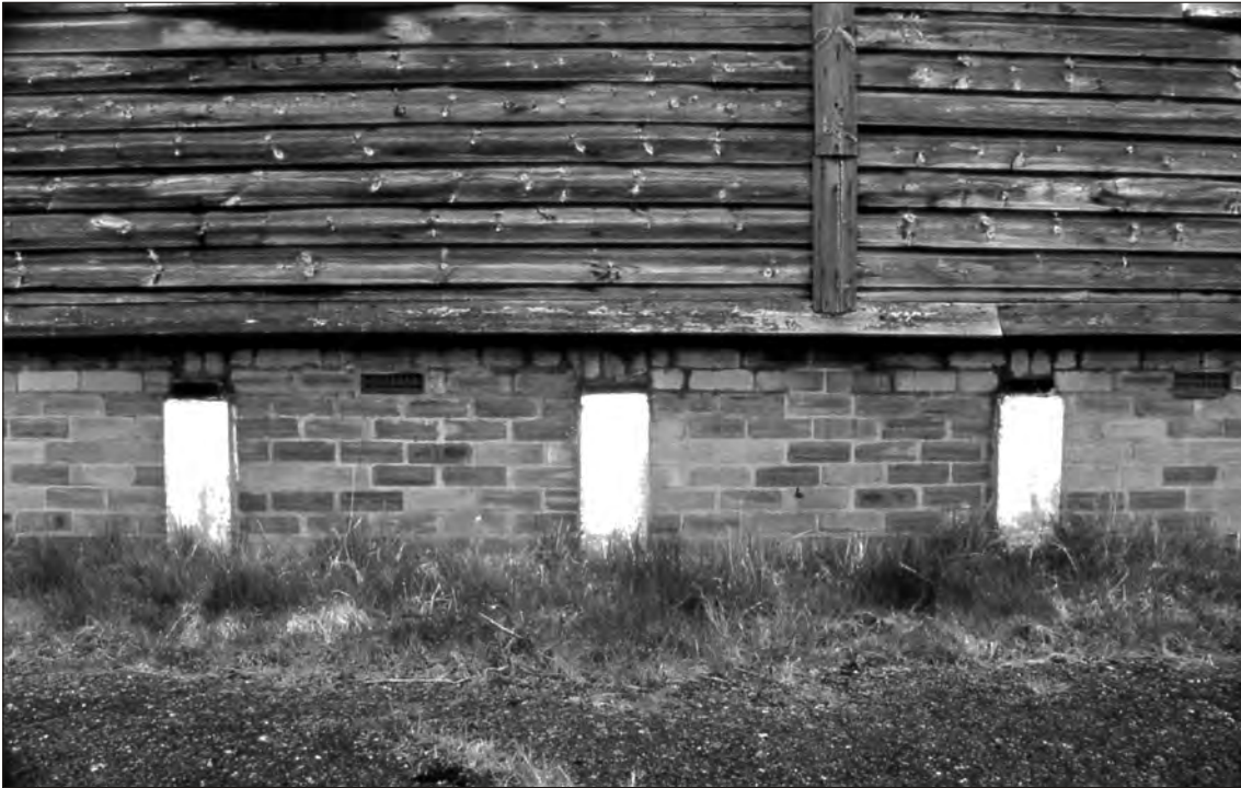
Plate 43 Saighton Camp, Chester: concrete foundation pillars in spider block 22 (also evident in blocks 21, 23 + 39); showing evidence for spider blocks having been raised off the original concrete foundation pillars.
